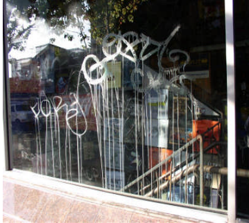
Before Acid Graffiti Damage
